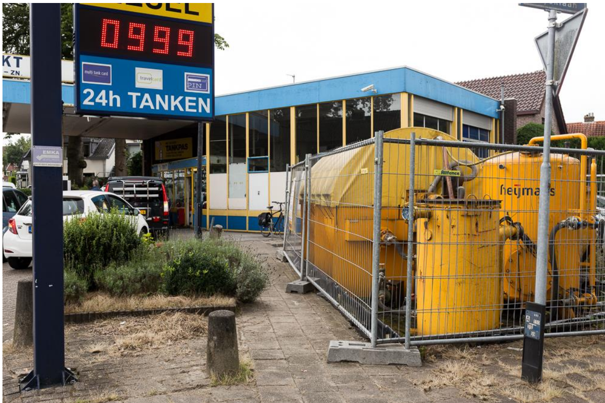
De Birk 6: 35mm, f/8, 1/40s, ISO100 – Today “De Birk” is the only gas station pricing diesel less than one euro per litre. The installation for soil sanitation is cleaning up a spill caused by leakage.
