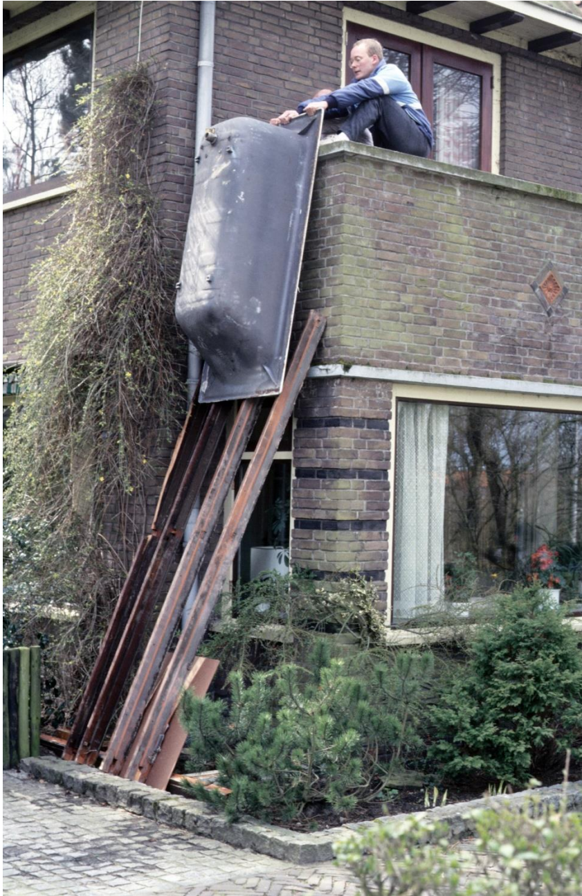
Family album 4: During the renovation of the bathroom, my father and I transport the old bathtub down (1980s)
